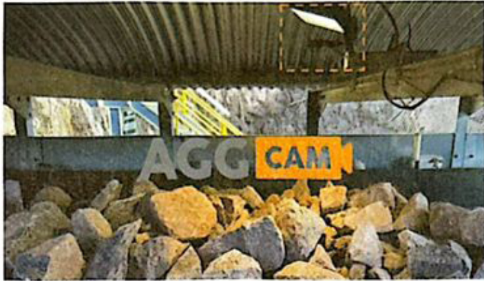
Mounsthorrel AggCAM installation above the CV1 conveyor belt
